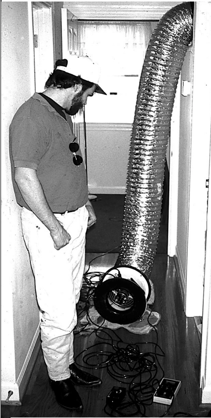
Connecting the duct blower to a single central return gives an accurate airflow reading as long as the ducts have been sealed to specifications listed in Chapter 5.
